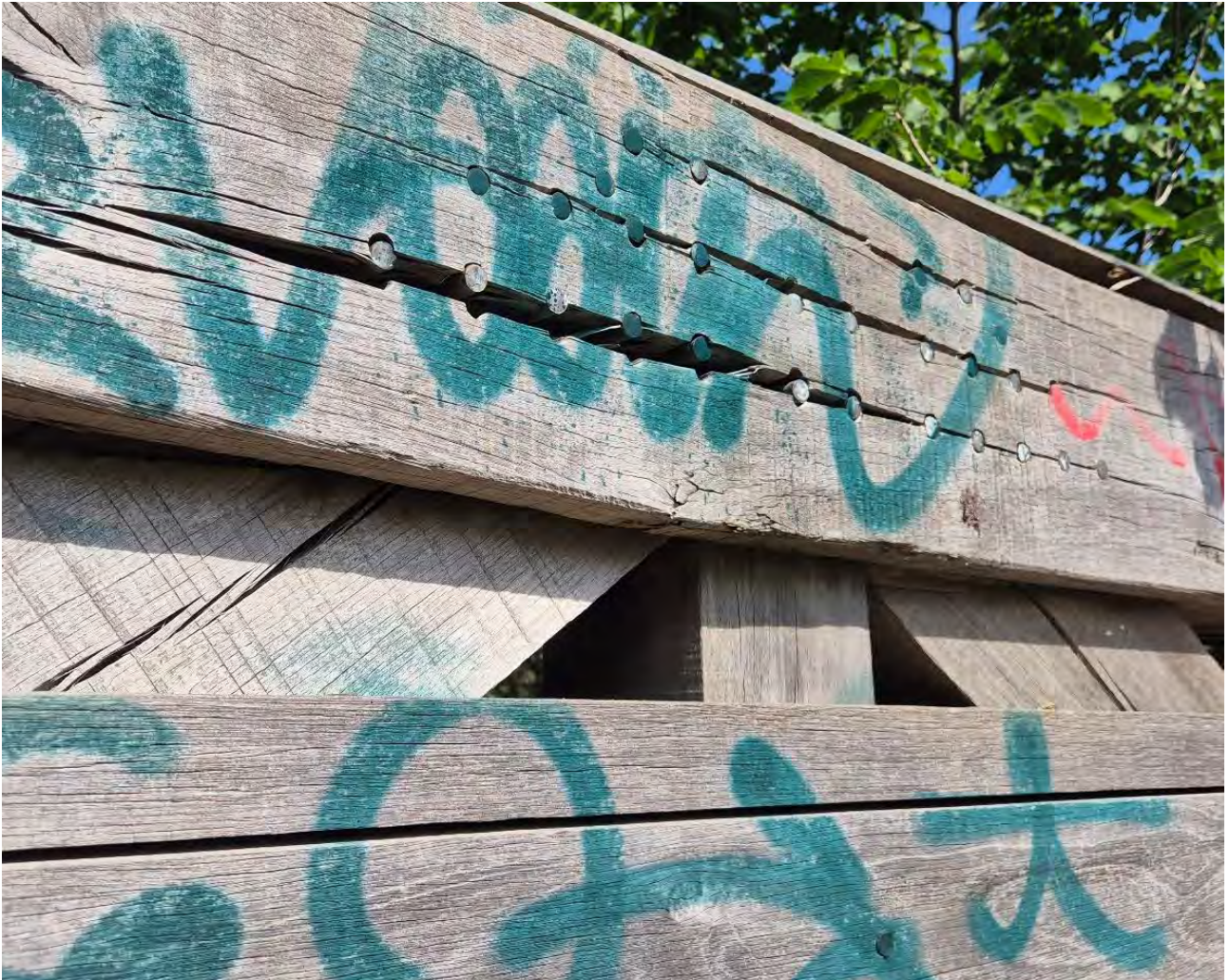
Figure 1: Top chord node – severe splitting in all members. Note right-hand diagonal displacing up and left-hand diagonal pulling down
